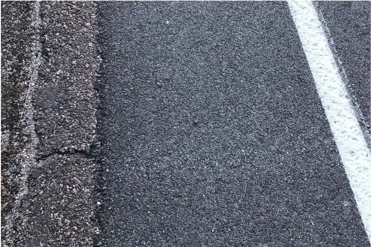
Figure 19. Transverse Crack in Shoulder at Approximately MM266.30
